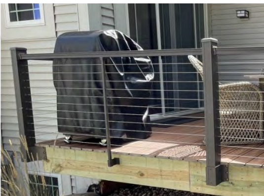
Townhouse Unit with a cable railing mounted on fascia (photo: Badgerland Exteriors)
