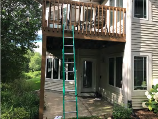
Ranch Unit with upper deck and lower concrete patio, (shown in old color) (photo: Siebers)
